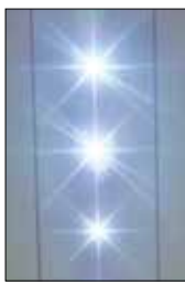
LED spots in the ceiling
