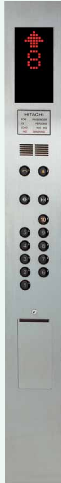
Operating panel (OPS-A98-1)
